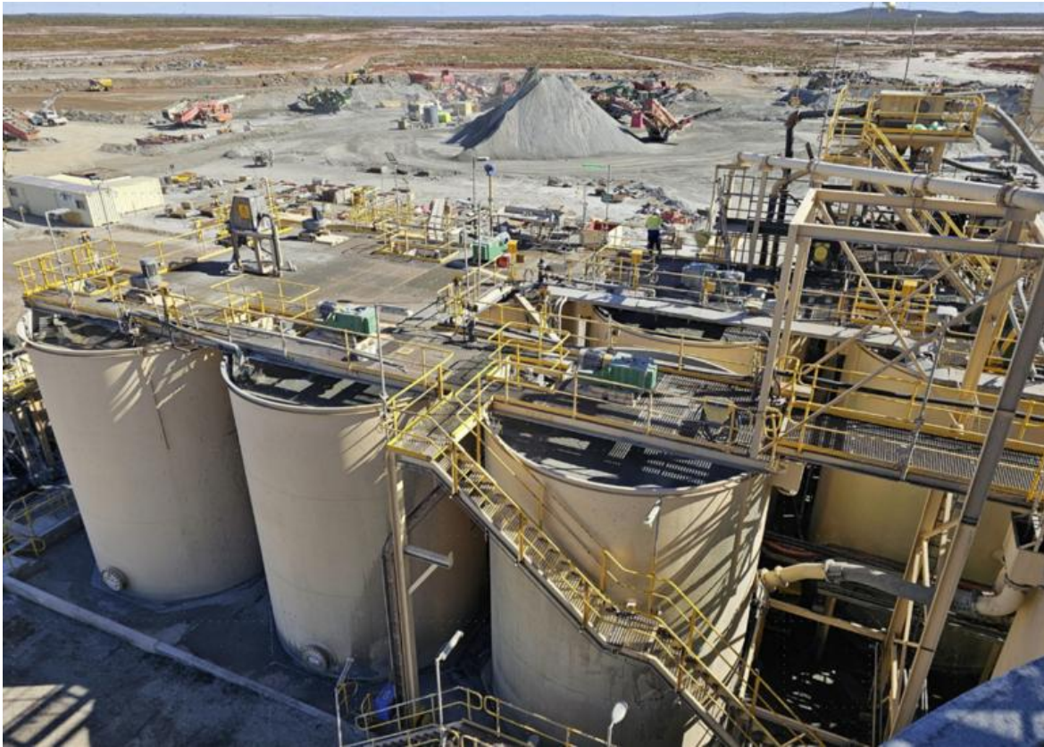
Figure 1: Lakewood Processing Plant
